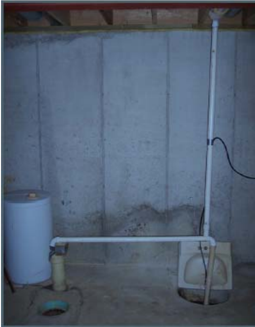
FOOTING DRAIN PUMPED INTO SANITARY SEWER
