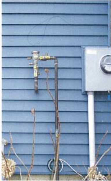
LAWN SPRINKLING PRESSURE VACUUM BREAKER
